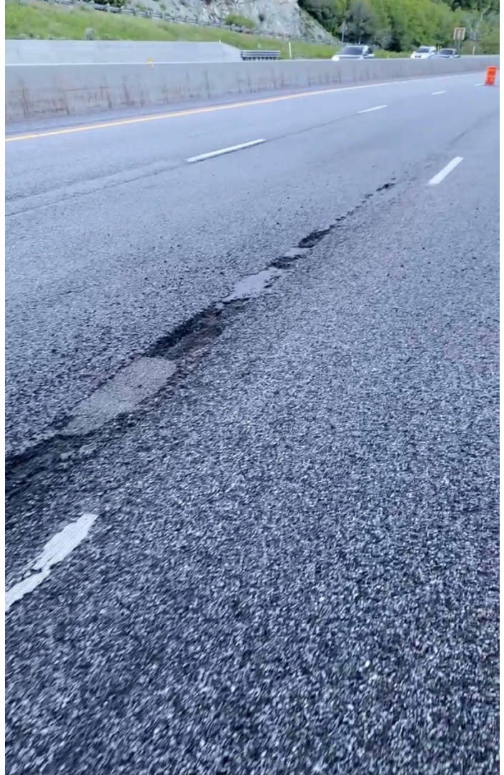
This paving seam has started unraveling and has created large potholes. The distress was cleaned with an air compressor in preparation of Mastic One application.
