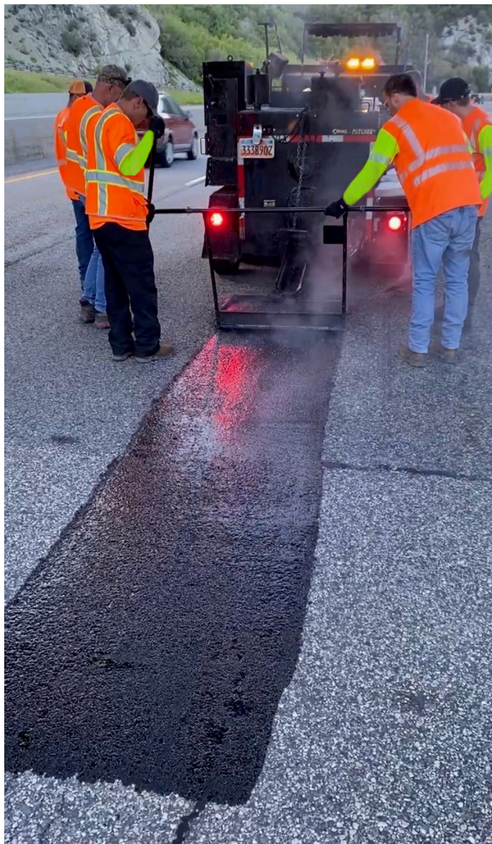
UDOT is applying Mastic One with a drag box to create a uniform application that is flush with the existing pavement. The aggregate in Mastic One is filling the distress voids to add structure and stability back into the pavement.
