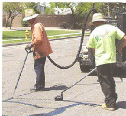
Effective treatment of cracks will help keep water out of the underlying pavement layers.
