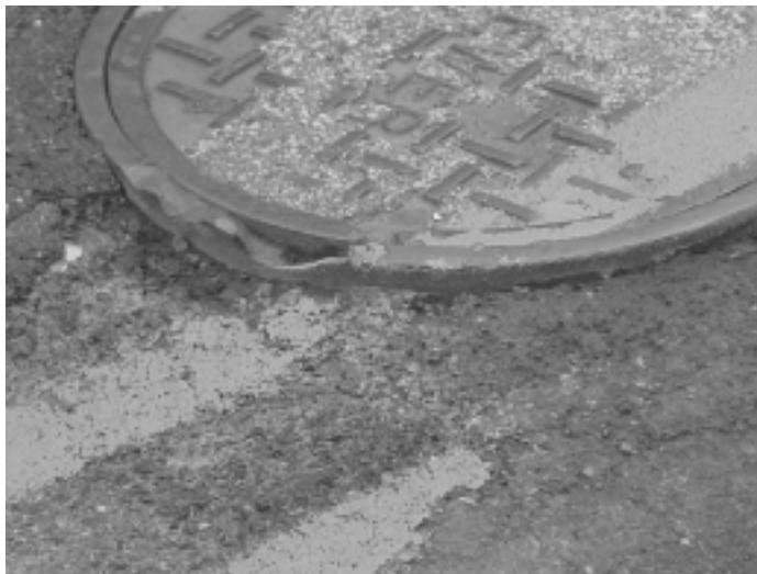
Manhole prior to treatment: not only snowplows suffered damage.
