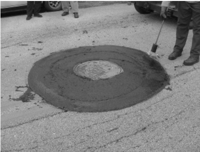
Torching the edge of a finished patch to seal it to the pavement.
