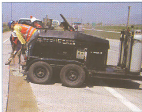
TechCrete was chosen in part because it can expand and contract with the pavement movement.
